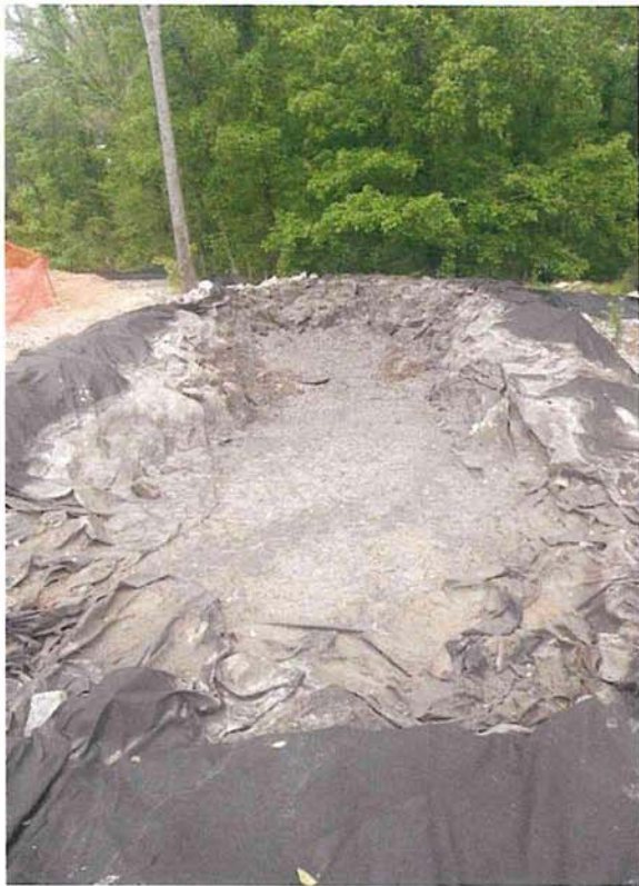
Inside of berm around MH 1750 before cleanup
